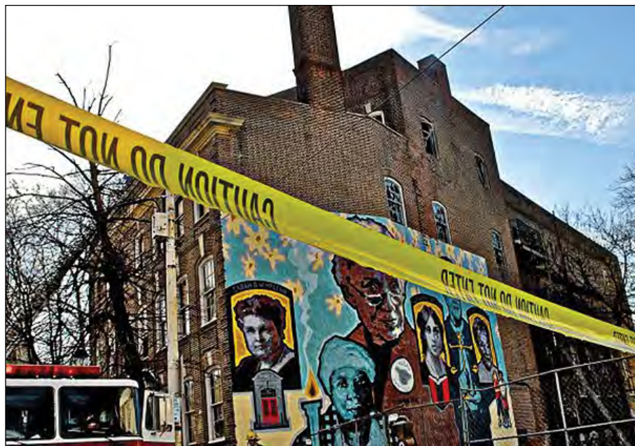
In 2012, fire ripped through this vacant and unsealed building, causing severe damage. It was owned by the Philadelphia Redevelopment Authority at the time.
