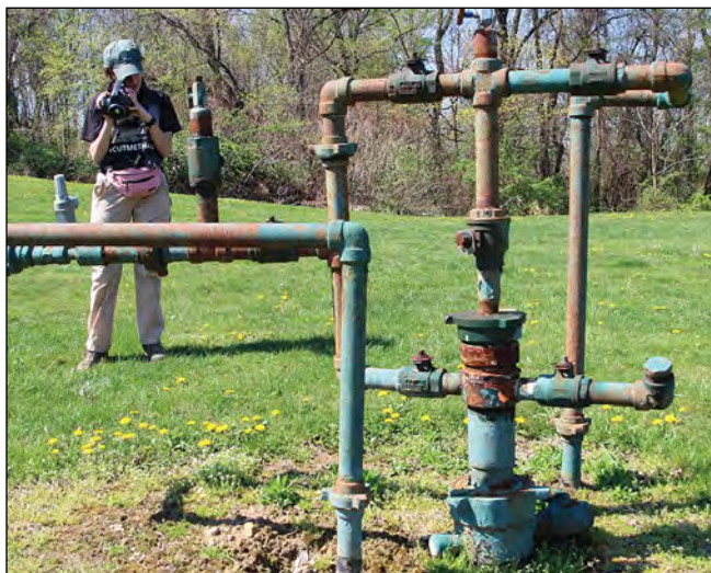
Melissa Ostroff, a licensed thermographer for the environmental group Earthworks, used an infrared camera to detect methane leaks from a natural gas well in Pennsylvania.
